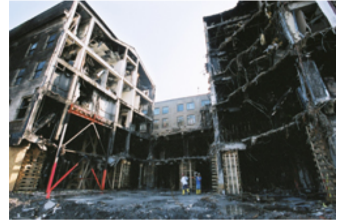
Arlington, VA, September 21, 2001 -- The exterior of the Pentagon crash site is shown after the area has been stabilized by shoring structures. (Photo by Jocelyn Augustino/ FEMA News Photo)
